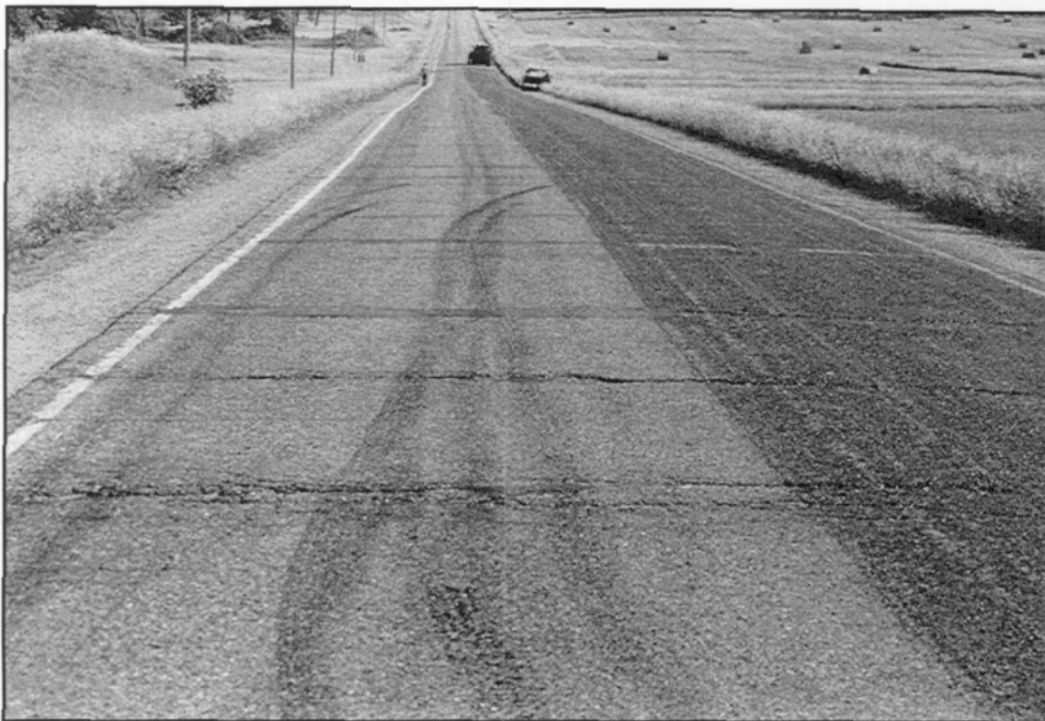
Figure 2. Typical Pavement Condition of T.H. 25 Before It Was Overlaid
